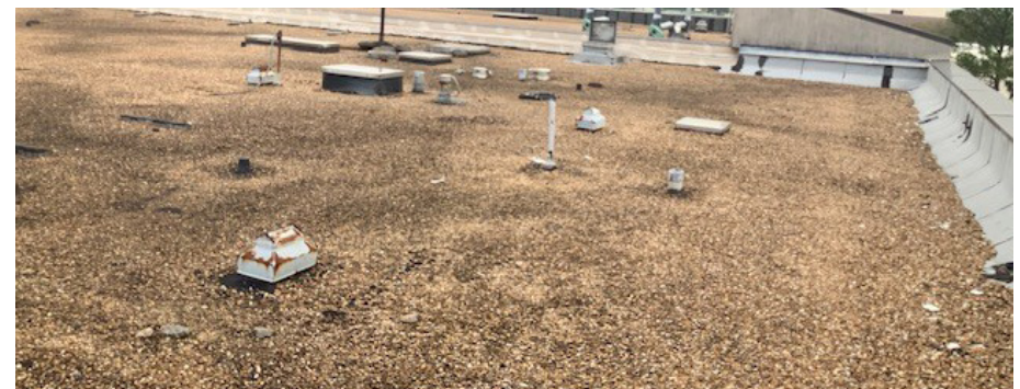
Roof replacement will be needed
