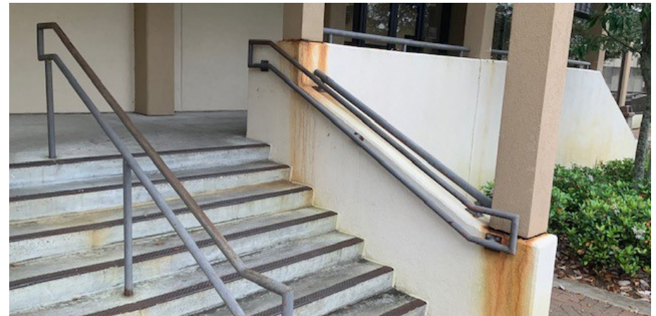
Evidence of water infiltration at base columns
